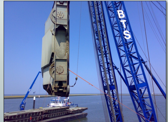
Waddenzee (Kornwerderzand) lock gate axles, coated with Lunac 2+ (2005)
